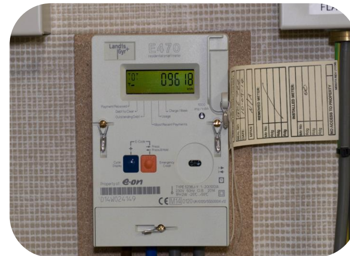
E-Meter (backup battery)
